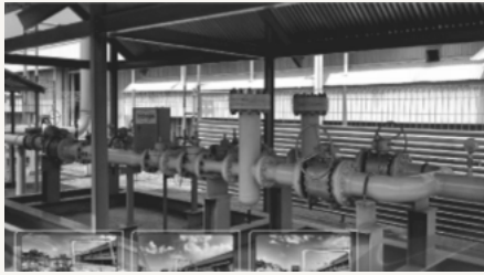
Fasilitas pipeline IKD, Wunut · IKD pipeline infrastructure
